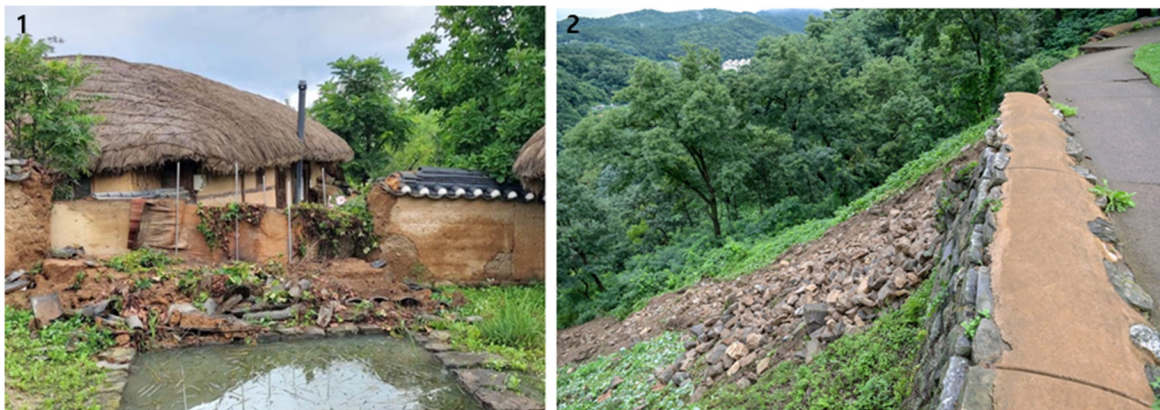
Fig. 1. Damaged cultural heritage due to heavy rainfall in 2020. (1) A collapse of the wall in the Andong Hahwye Village, (2) A collapse of the fortress wall of the Gongsanseong Wall
